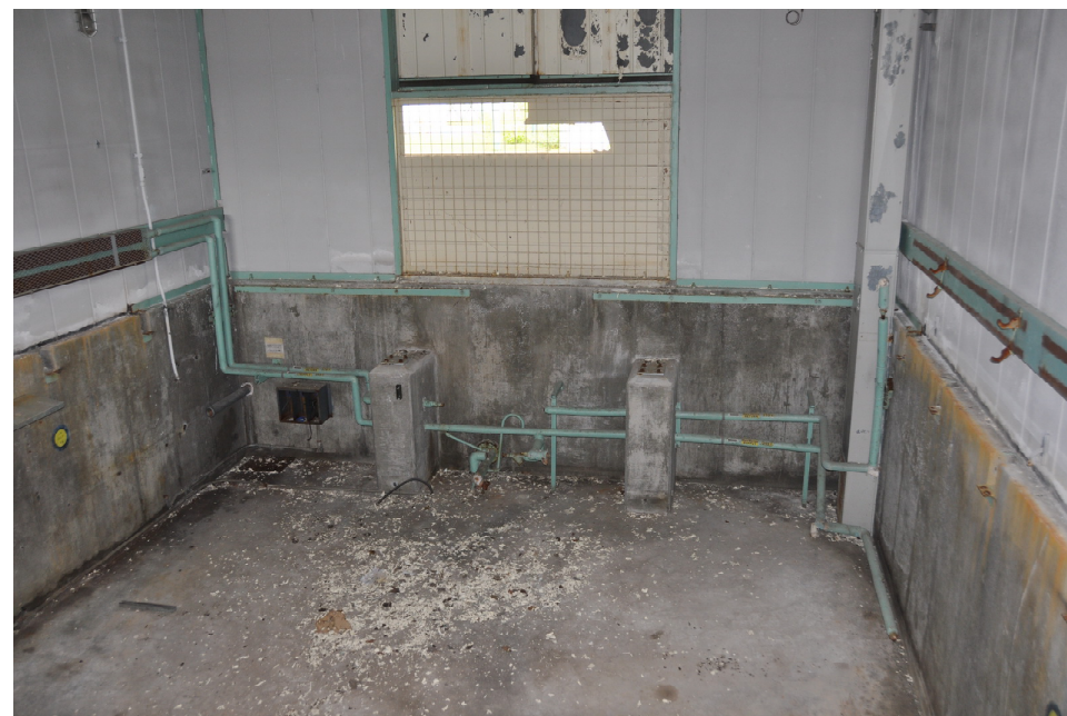
Below, a view into the pit. Note the columns at the back which supported the launcher and above them, the blow-out panel.
