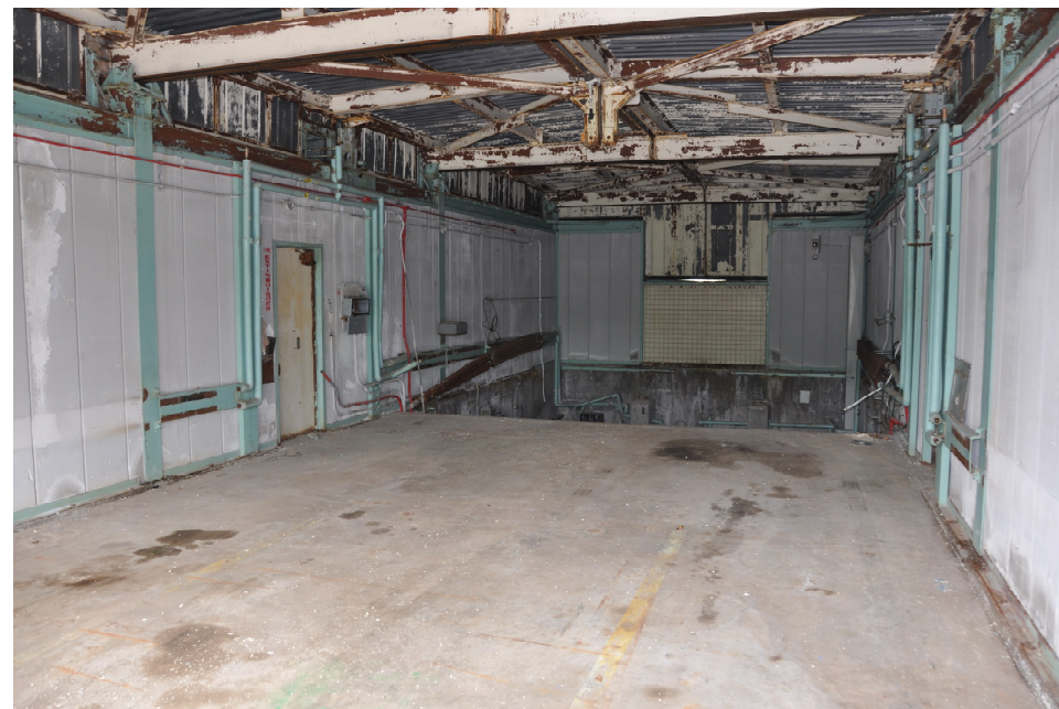
Above, a view inside the decommissioned shelter. Note the pit in the back of the shelter. The area around the launcher was covered with a steel grating.
